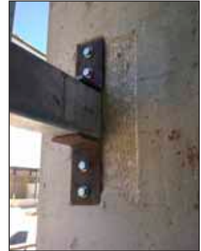
Titen® HD screw anchors were used to retrofit the Kalwall window frame openings
